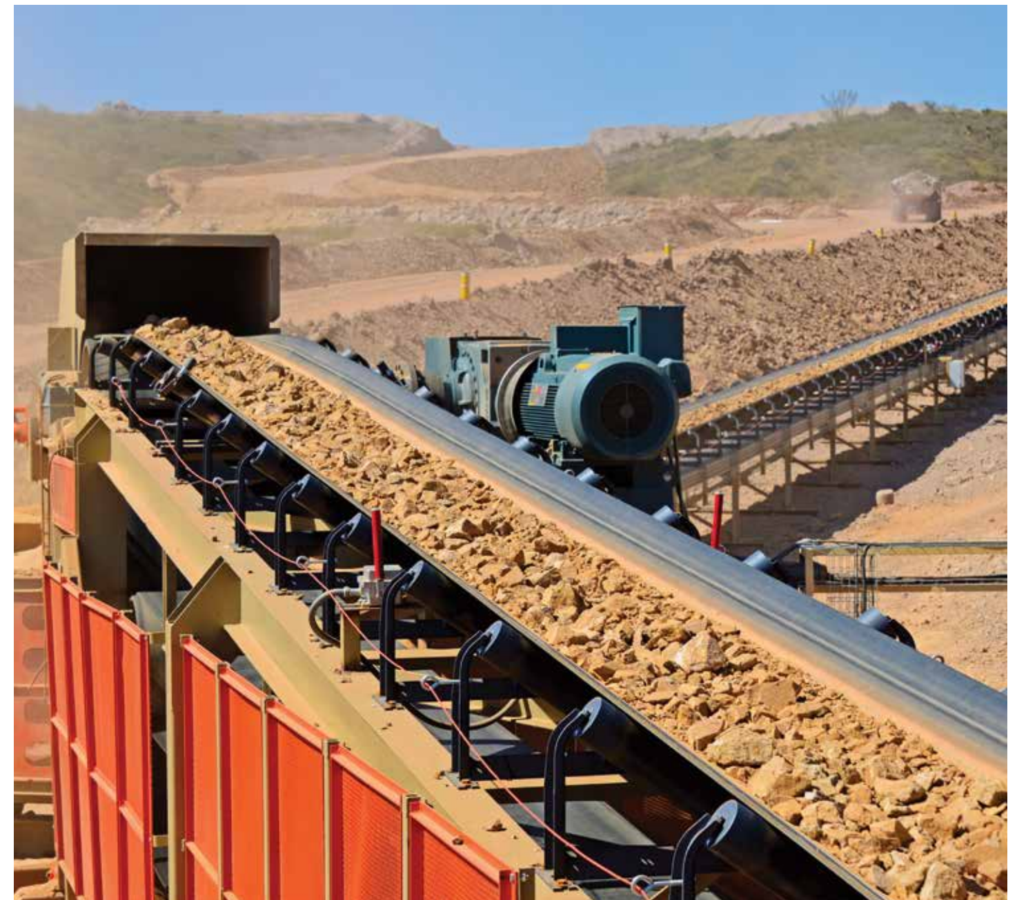
Due to the sheer scope of the project, the OEM wanted to partner with one supplier that could not only provide all of the components, but could also offer mining industry expertise and engineering support. According to mine officials, El Castillo’s overland system – powered by Baldor products – is working well, and they are pleased with the project.
