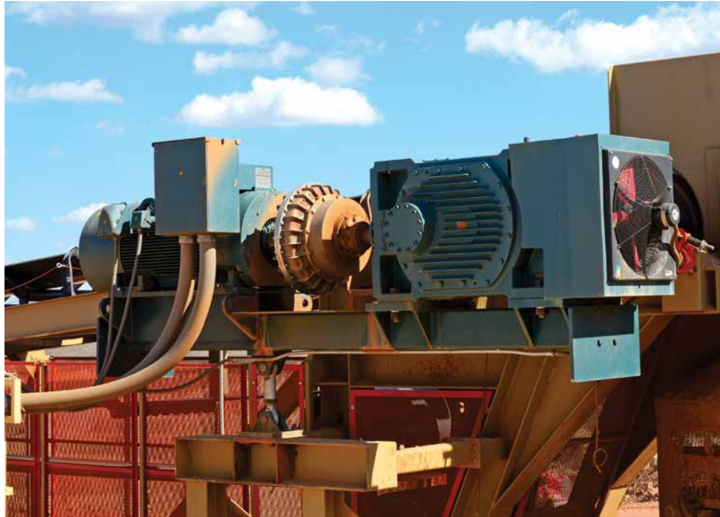
Mine officials wanted a packaged solution that would provide a smooth, soft start but was also powerful enough to pull a heavily loaded belt up 1,890 feet with a 226-foot lift. The solution: a Baldor•Dodge® MagnaGear® right-angle reducer and a custom 500 HP Baldor•Reliance® motor with an integrated backstop, mounted on a heavy-duty swing base. A Baldor•Dodge fluid coupling provides the soft start. The rest of the Baldor•Dodge package includes a custom-engineered moment coupling, MDX® pulleys and bearings.
